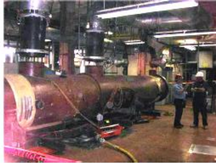
After inflating the air casters, the 40 ton heat exchanger moves easily across the factory floor to meet the crane.
