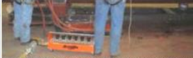
An orange AeroGo Load Module is inserted beneath the feed water heater. The control console box in the foreground regulates air into each of the individual Load Modules.
