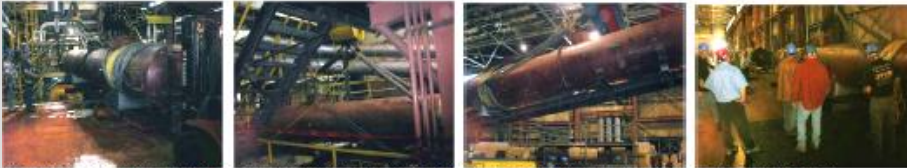
Still resting on casters, the heat exchanger is suspended over 9 stories, then successfully lowered to the floor without incident.
